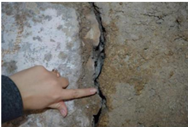
Figure 18 Vertical Structural crack inside the Mosque
