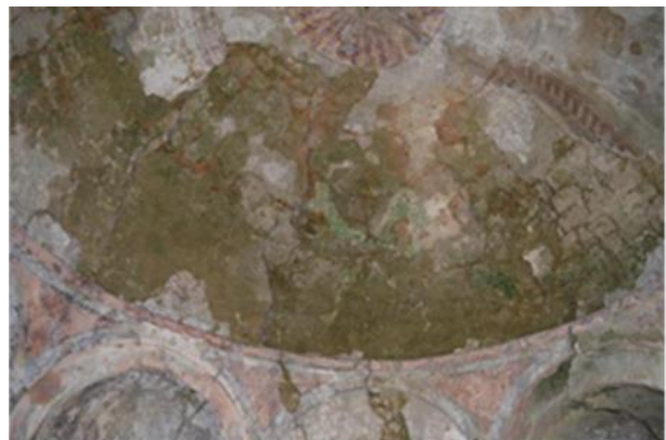
Figure 19 Structural cracks in the dome of the Mosque
