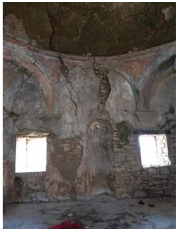
Figure 21 View of the dome and the vertical structural cracks from the inside
