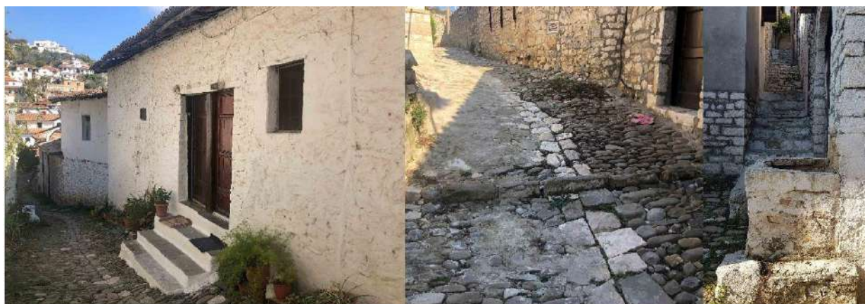
Figure 35. Surrounding walls facing the road, inappropriate or damaged doors, damaged or cumbersome road cobblestones and unsuitable concrete elements.
