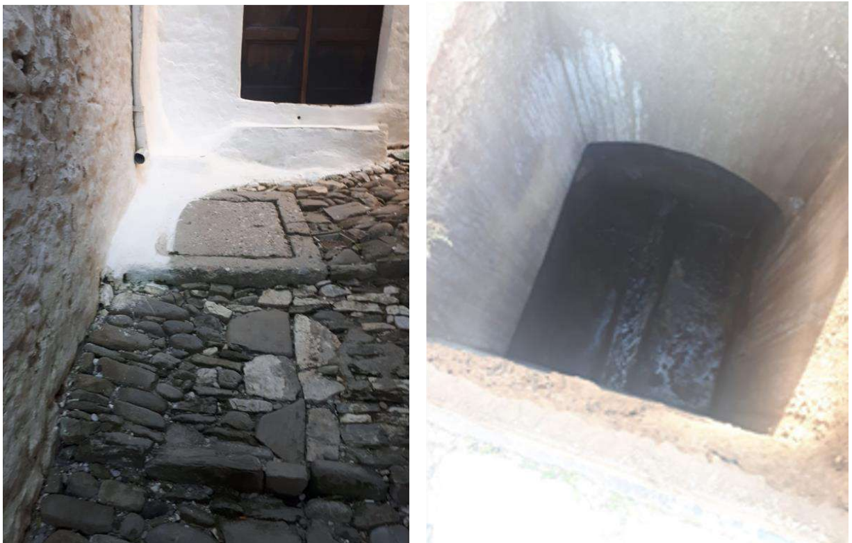
Figure 31. Waste water sewage network
