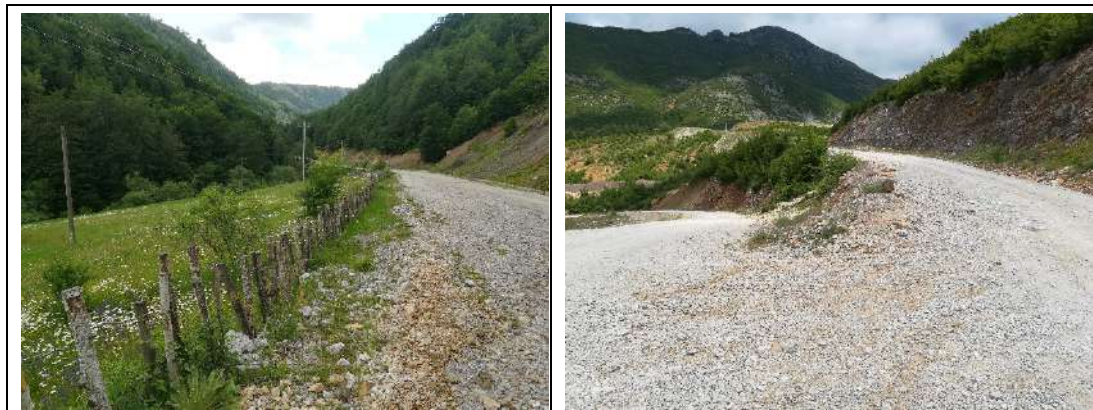
Figure 1-1: Examples of sections of the road in Fushe Studen (left) and Lunik (right)
