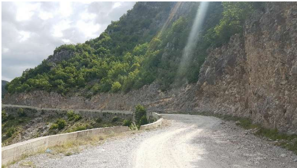
Figure 4.20: Photograph of the Zgosht to Cerenec road at shkembor lart kanion Poshte, approximately 35 m from the western border of the Shebenik-Jabllanicë National Park. The steep sided hill cutting and retaining wall have fragmented the forest habitat and are likely to serve as a barrier to the movement of some fauna species (444165.84, 4569530.41).
