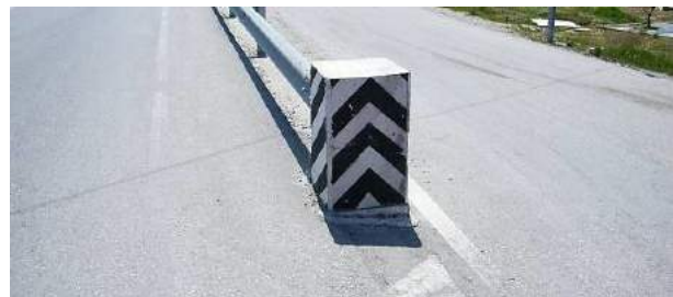
Dangerous “end treatment”- concrete block
