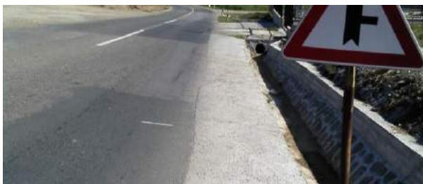
Unsafe drainage system, with headwall
