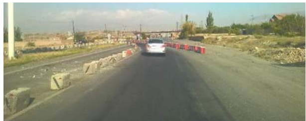
Dangerous work zone
