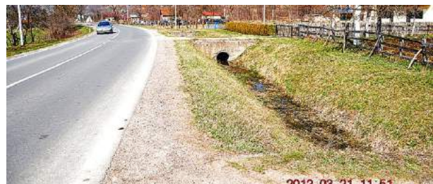
Unsafe drainage system, U-Type with headwall
