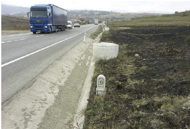
This drainage system as an obstacle
