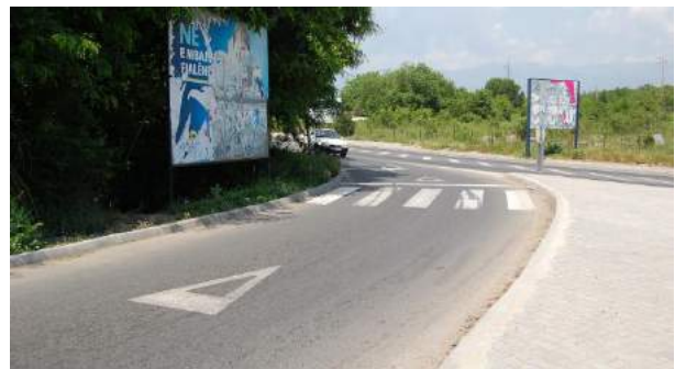
Missing of pedestrian footpath
