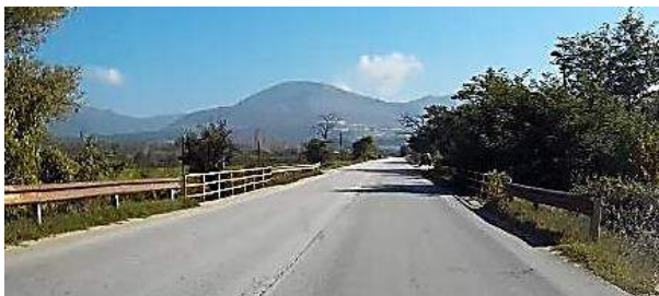
Dangerous guardrails (not a system)
