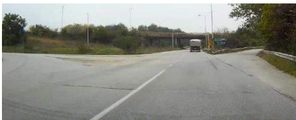
Missing channelisation in junction
