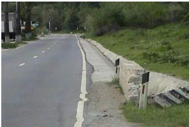
Unsafe headwall of a culvert
